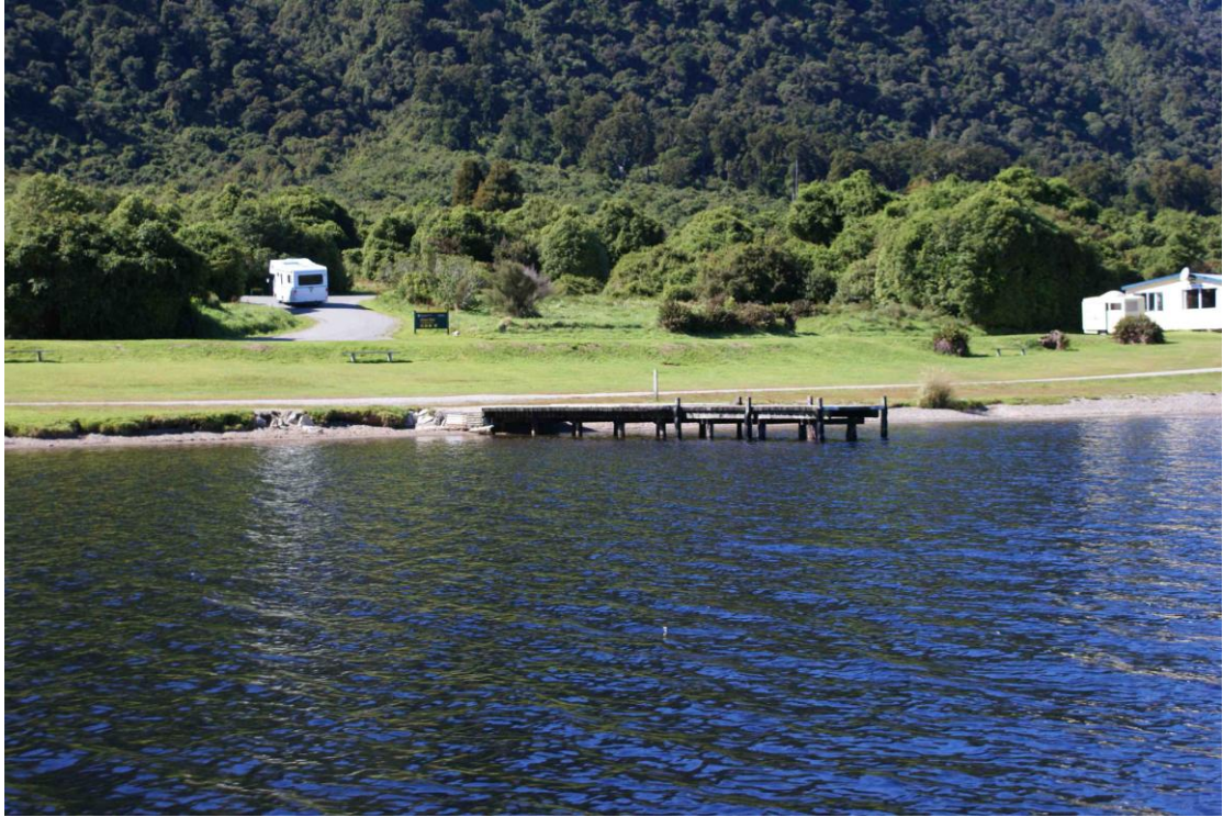
Figure 10 Erosion at the jetty at Hans Bay.
