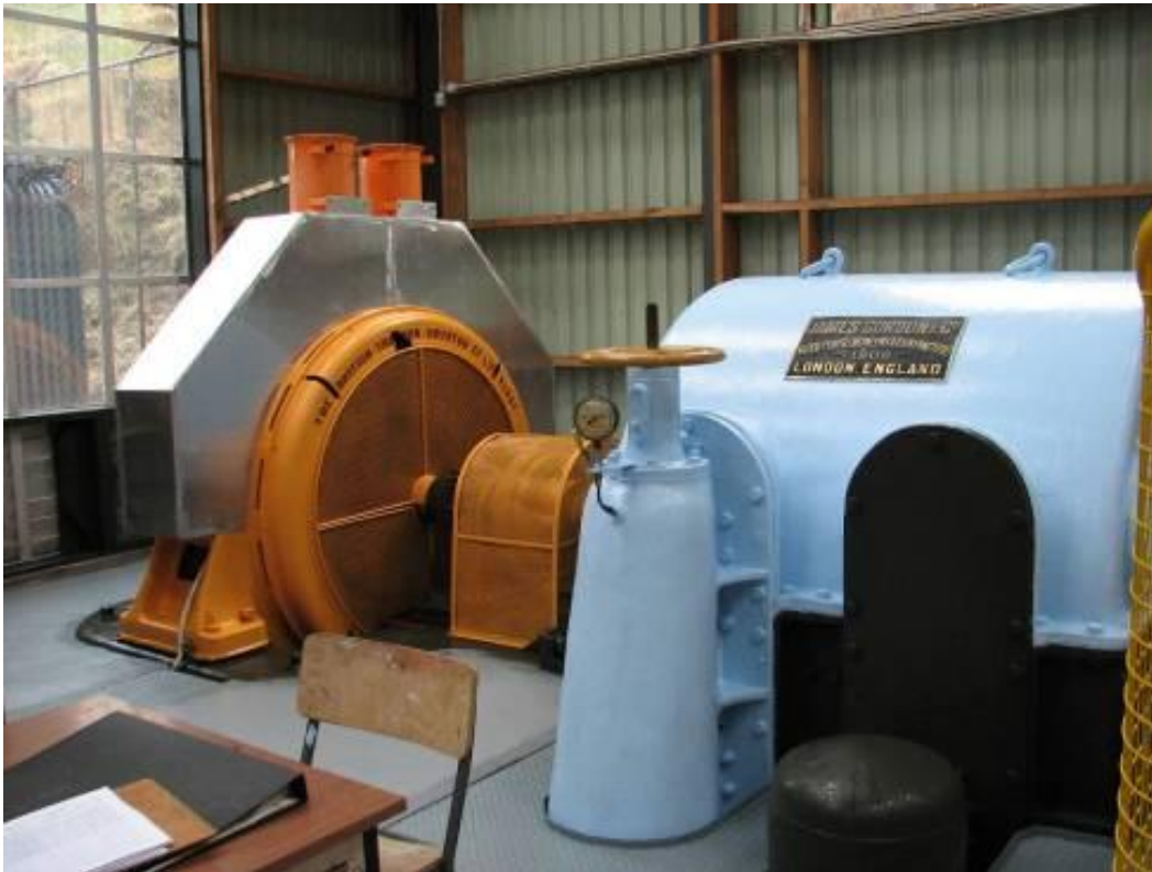
Figure 12. The original turbine and generator in the Kaniere Power Station
