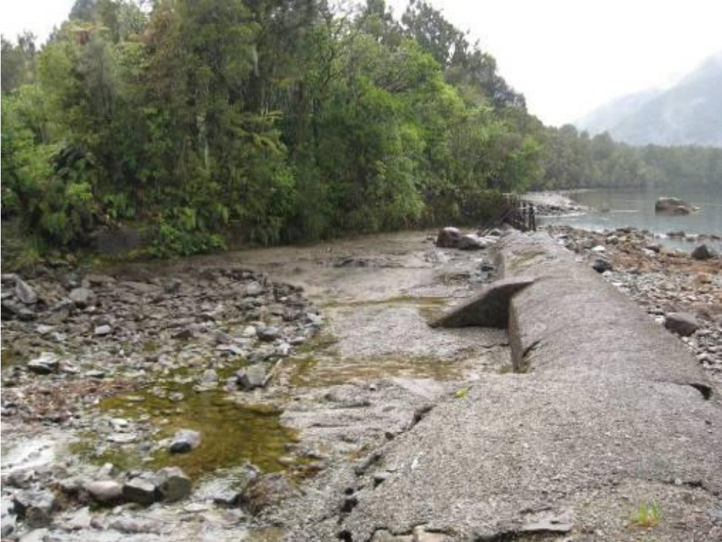
Figure 3. The 1916 concrete weir on Lake Kaniere with the possible remains of an earlier weir immediately downstream
