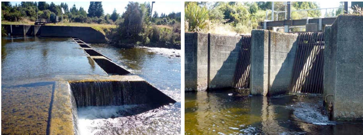
Figure 1.5 McKays weir (left) and intake to McKays race (right).
