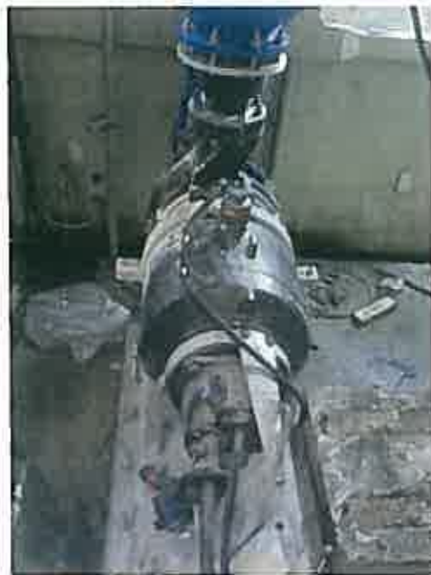
Fitzherbert Street Wastewater Pump Station – Pump Upgrade
