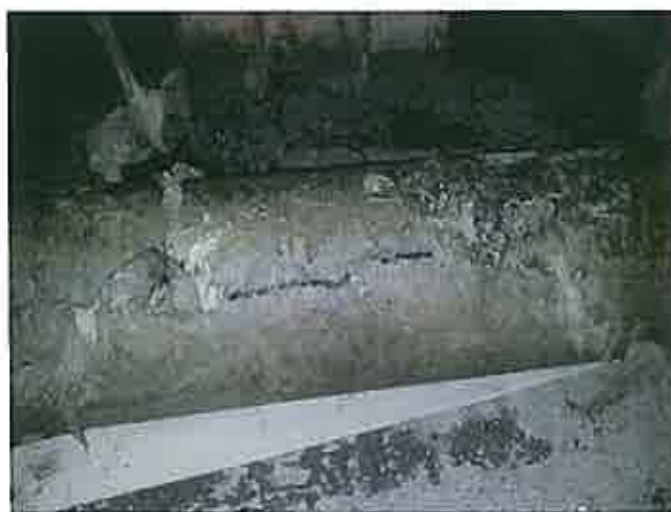
Hokitika Wastewater Pumping Main Split
