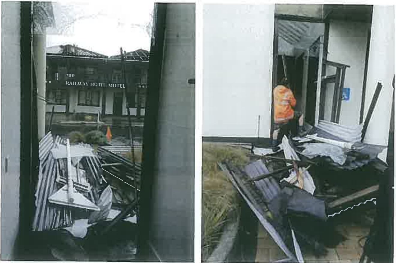
Headquarters Entrance – Tornado Damage
