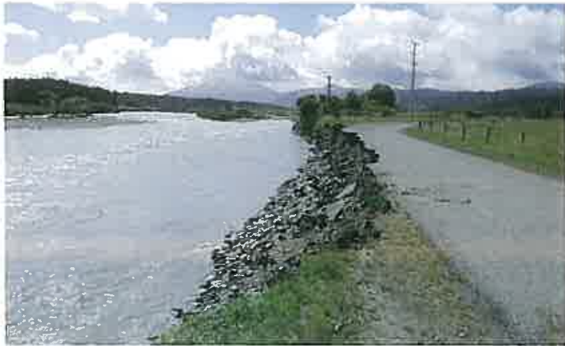
South Bank Arahura Road – Road Washout
