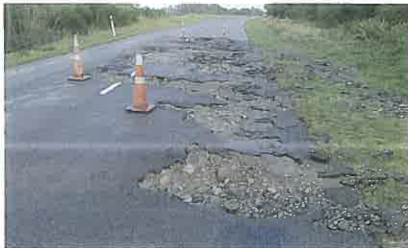
Kokatahi/Kowhitirangi Road – Carriageway Scouring
