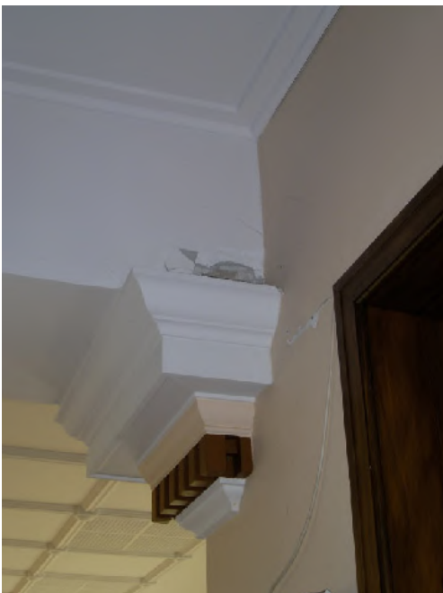
Photo 3 – Damage to the beam above the mezzanine floor prior to restoration works
