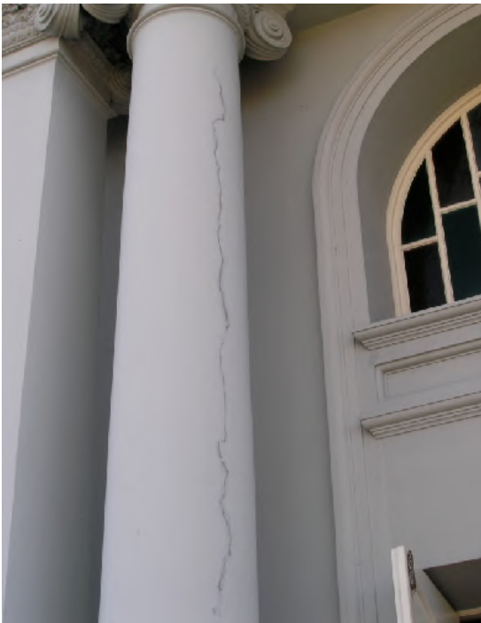
Photo 9 – External columns prior to the restoration works showing vertical cracks
