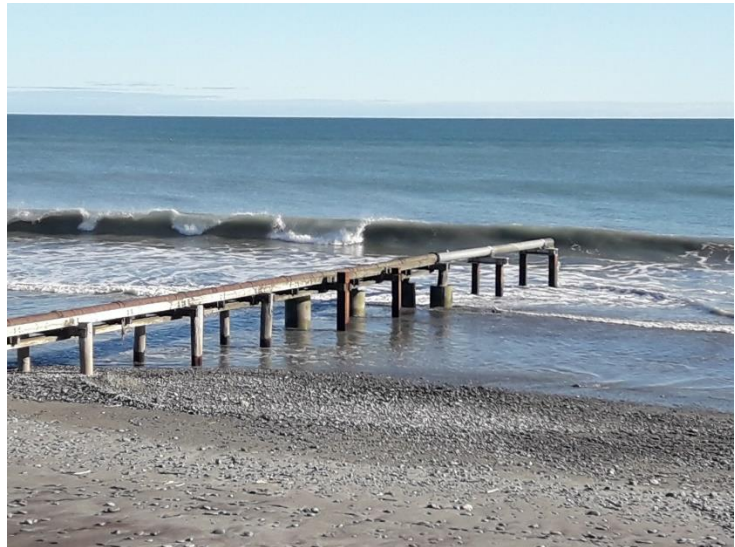
Figure 1-6: Treatment Plant Outfall.
