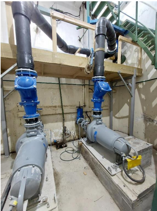
Figure 1-5: Fitzherbert Pump Station.
