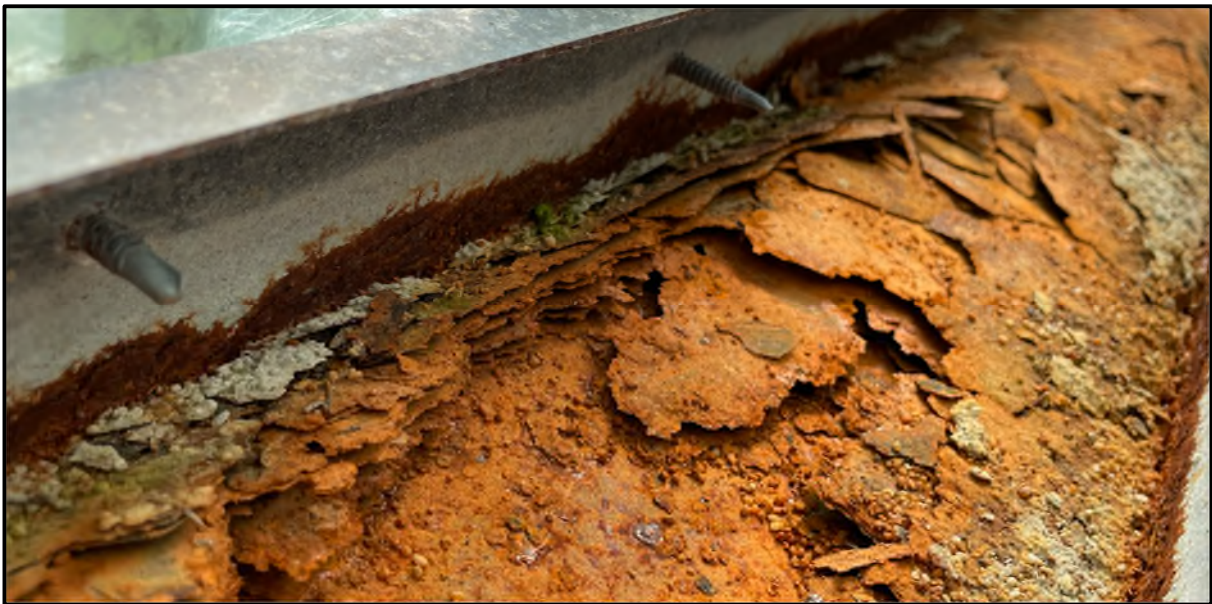
Photograph 7: Corrosion and Delamination of the Web to the Upper Girt Between Grid Lines 4 and 5
