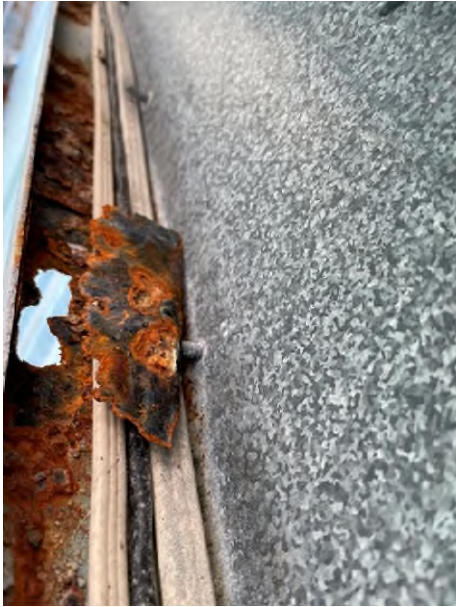
Corrosion to Eaves Beam Grid Line A
