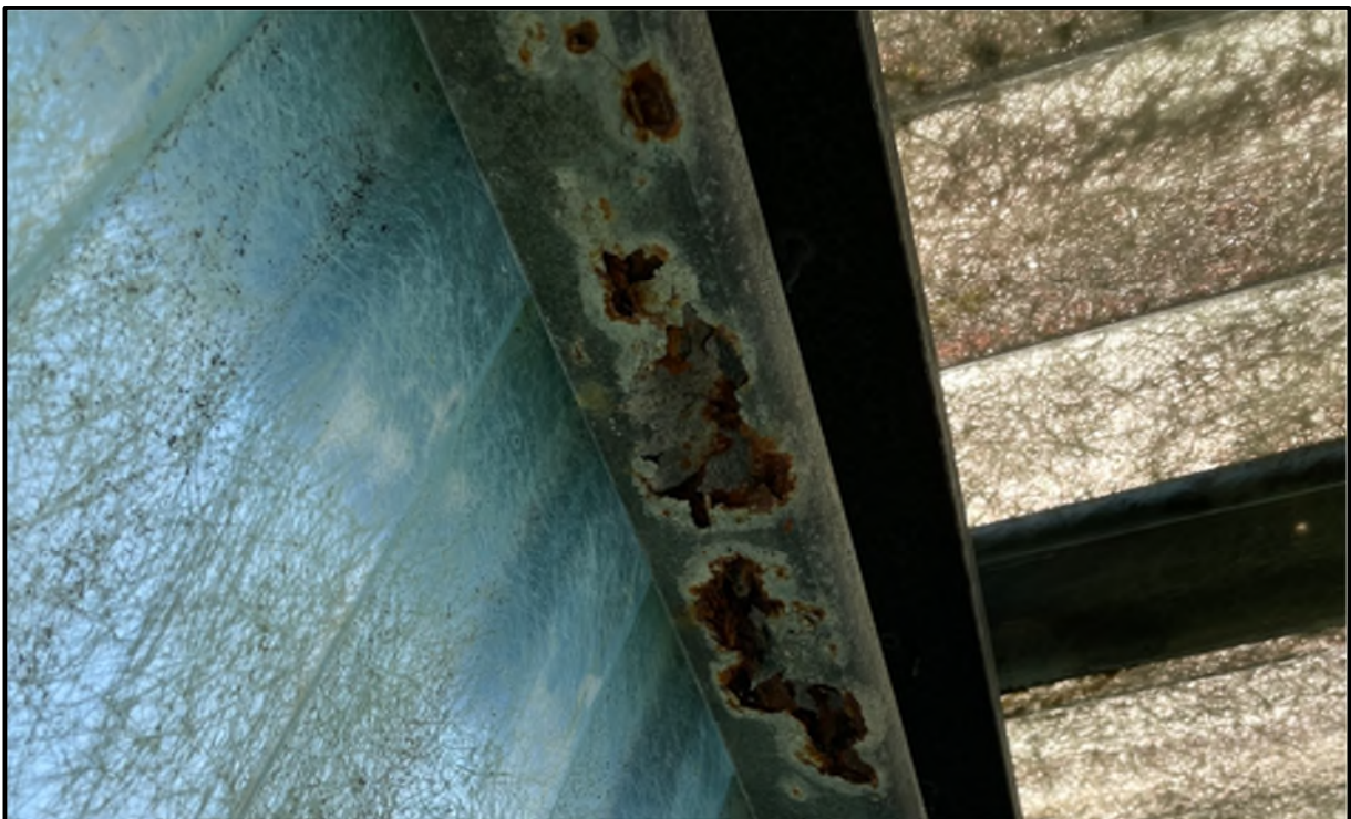
Photograph 9: Holes in Bottom Flange of Eaves Beam Between Grid Lines 6 and 7
