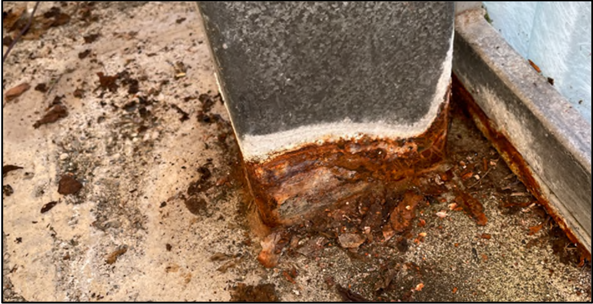
Photograph 6: Corrosion to Door Post Between Grid Lines 2 and 3
