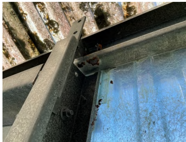
Corrosion and Hole through Eaves Beam Grid Line A
