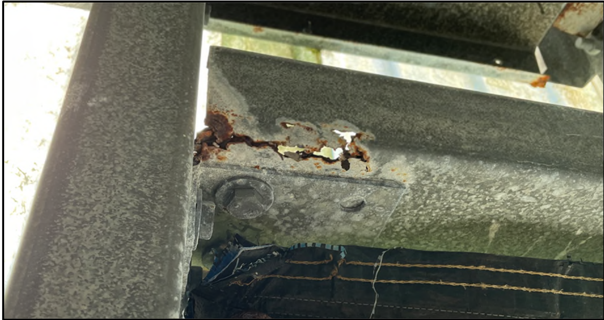
Photograph 10: Corrosion to Door Head Beam at Western End
