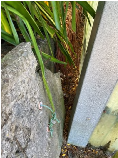
Gap Between Retaining Wall and South Elevation
