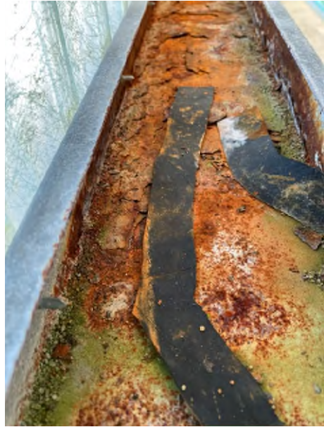
Delamination to Girt Grid Line A
