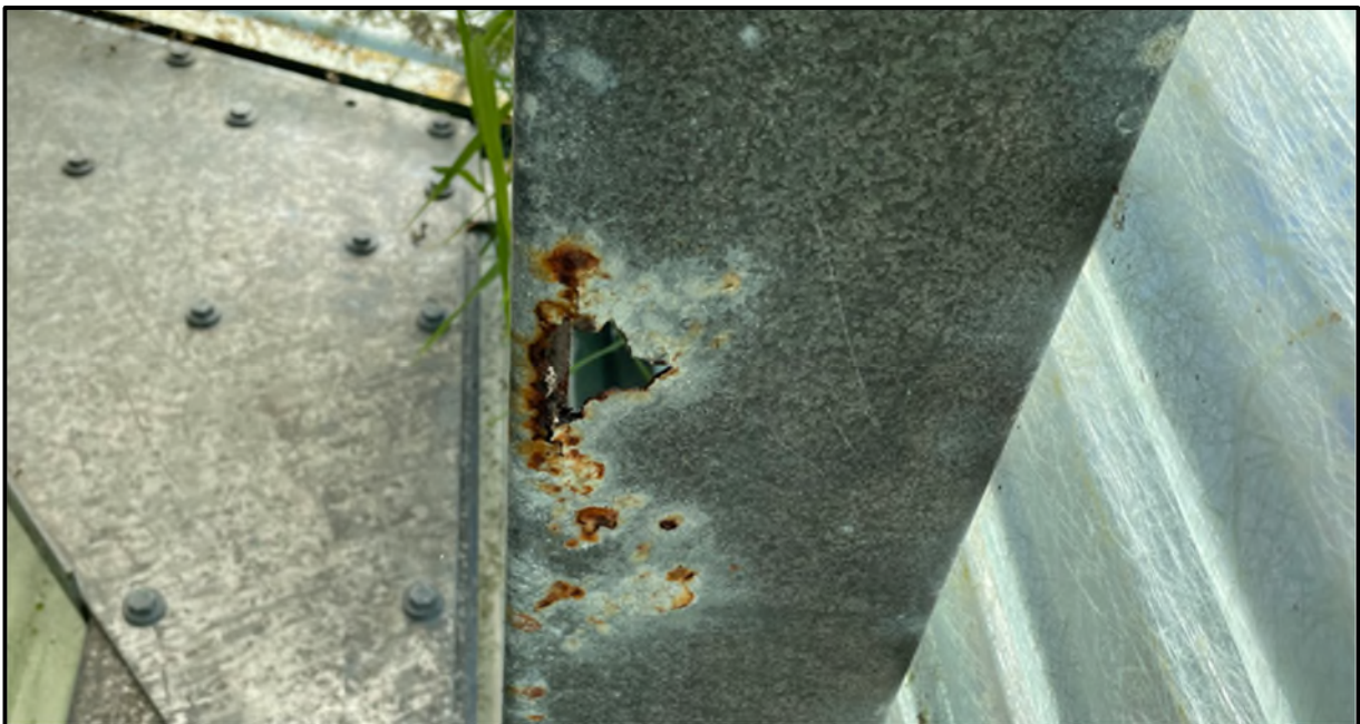
Photograph 5: Holes in Web of Girt between Grid Lines 1 and 2
