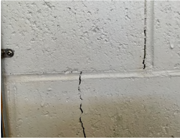
Paint Across Stepped Crack – Horizontal Mortar Un-cracked
