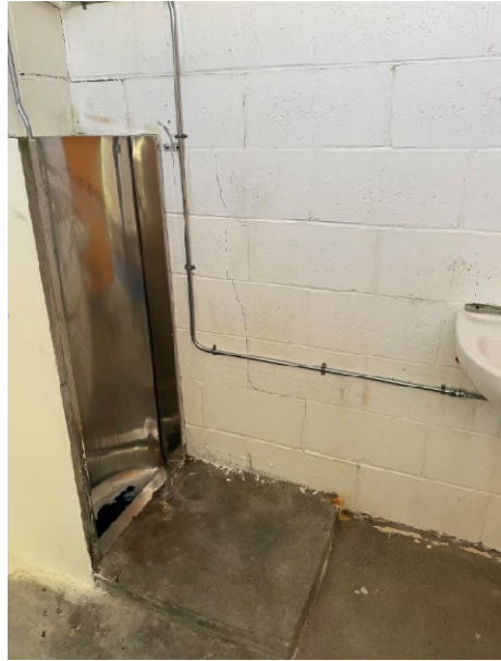
Stepped Crack in Concrete Masonry Wall – Male Changing
