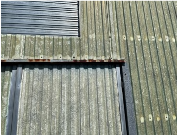
Corrosion to Flashing Over Door – North Elevation
