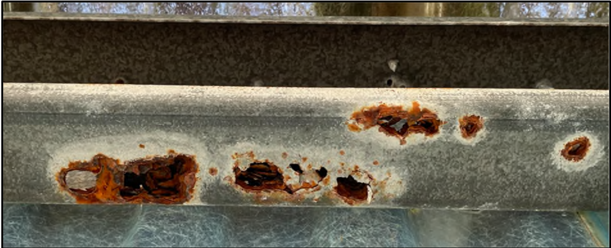
Photograph 12: Corrosion, Holes and Delamination to Eaves Beam, Grid Line 6 to 7
