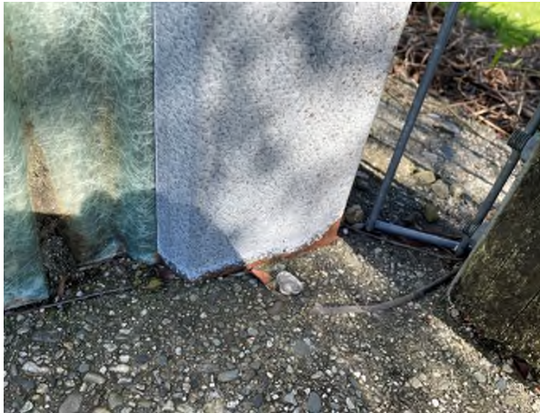
Corrosion, North West Corner
