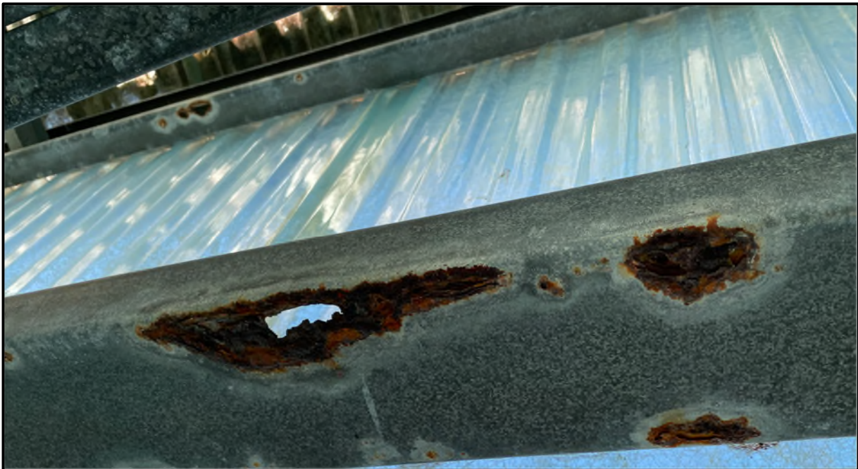
Photograph 14: Holes to both Upper Girt and Eaves Beam
