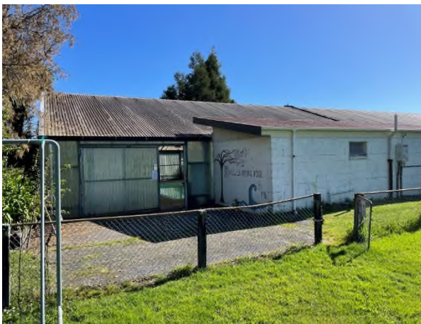
Vertical Crack Under Window
