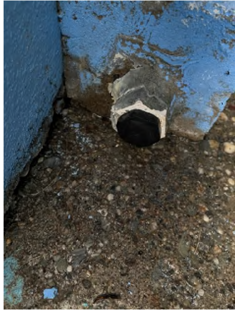
Leaking Valve to Paddling Pool
