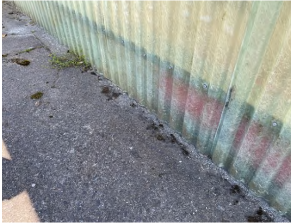
Cladding in Contact with Ground
