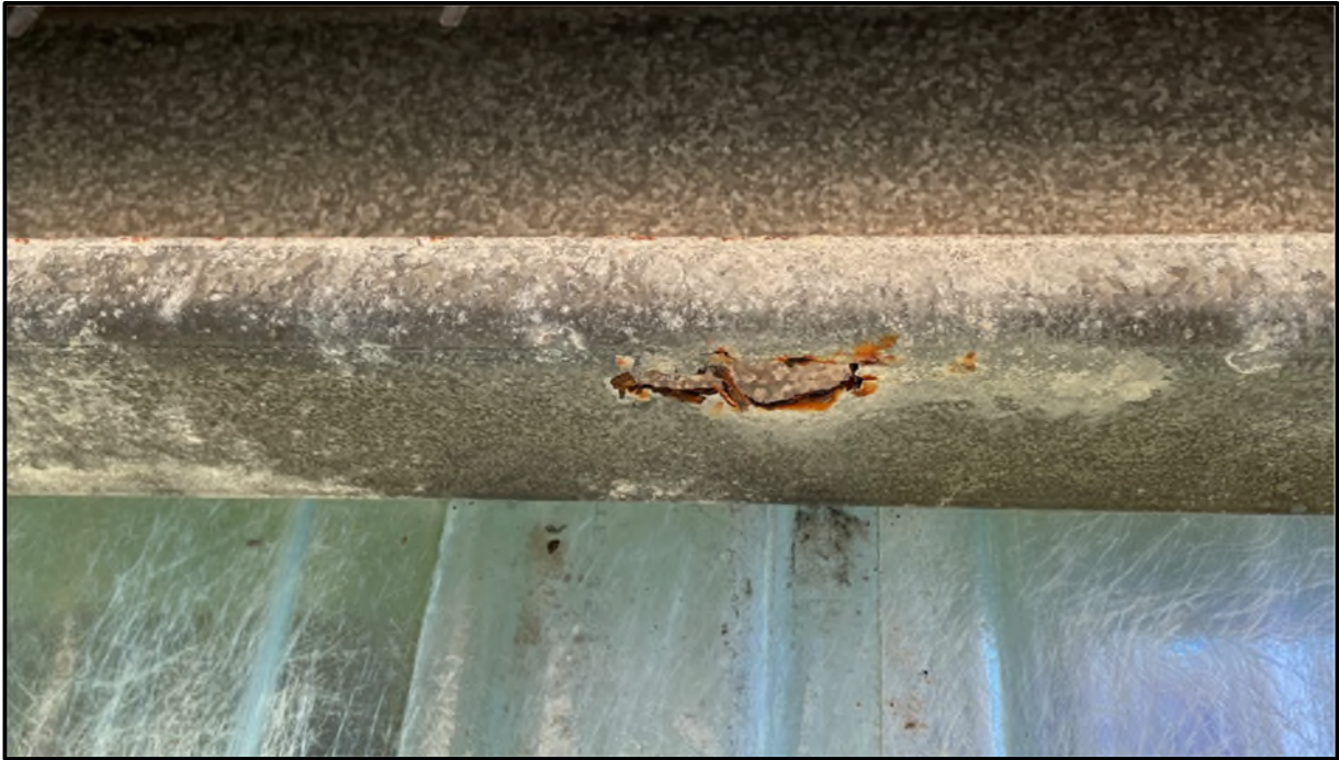
Photograph 8: Hole to Lower Flange in Eaves Beam Between Grid Lines 4 and 5
