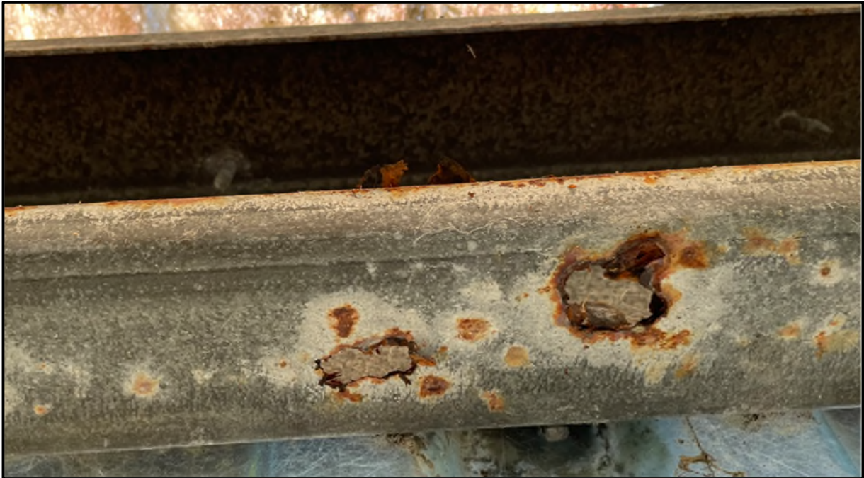
Photograph 4: Holes in Flange of Eaves Beam between Grid Lines 1 and 2
