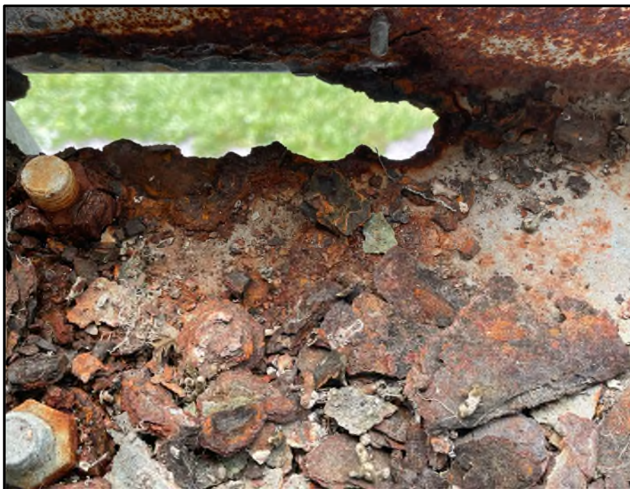
Photograph 11: Inside Face of Door Head Beam Showing Corrosion and Delamination
