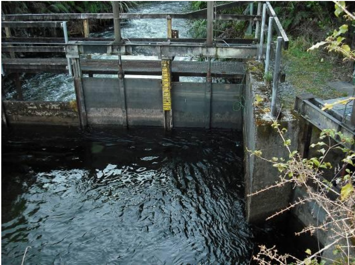
FIGURE 2.1.2 [CONTROL GATES TO KANIERE RIVER/MCKAYS CREEK (CENTRE) AND TO THE KANIERE FORKS RACE (RIGHT)]
