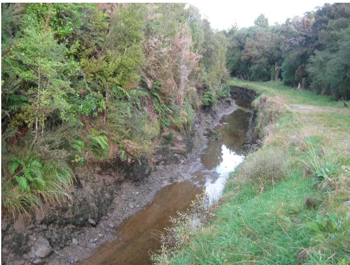
FIGURE 3.5.1 [MCKAYS WATER RACE FROM TUNNEL TO HEADPOND]
